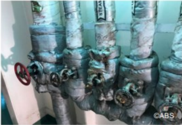
Handwheel missing, lagging damage
