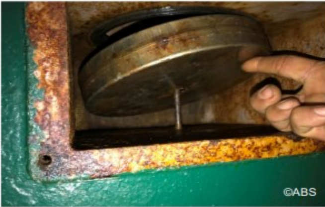
Tank vent disk wasted
