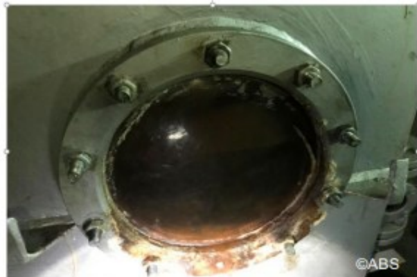
HT Water expansion tank sight glass leaking
