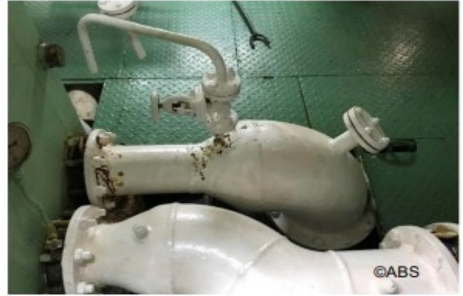
Main Fresh Water cooler inlet pipe leaking
