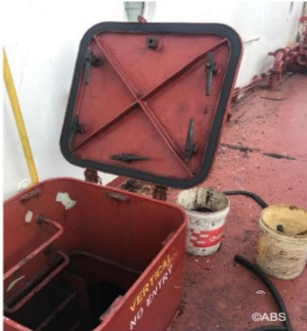
Missing Dog for watertight hatch cover
