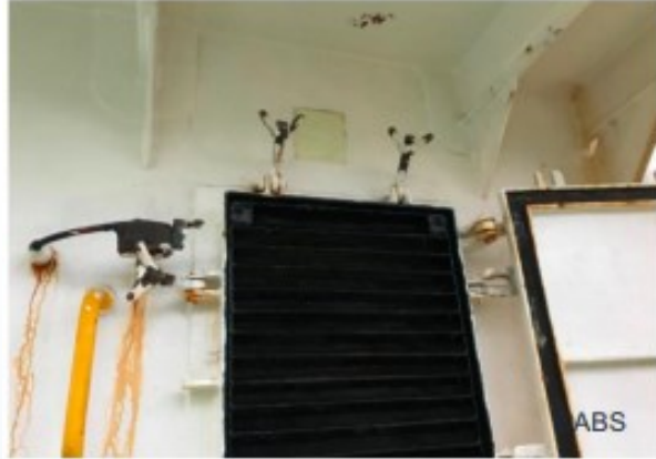
Watertight indication sensor not operational
