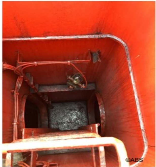
Loose/broken lighting inside vertical trunk
