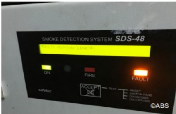
Cargo Hold Smoke extraction system faulty
