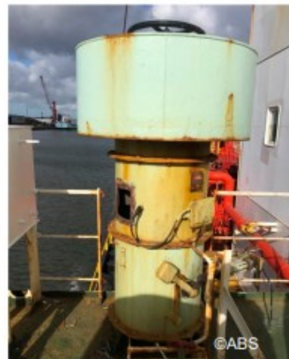
ER ventilation fan damper unable to operate
