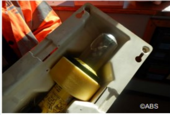
SART located in Bridge with shell cracked, and damaged and not watertight
